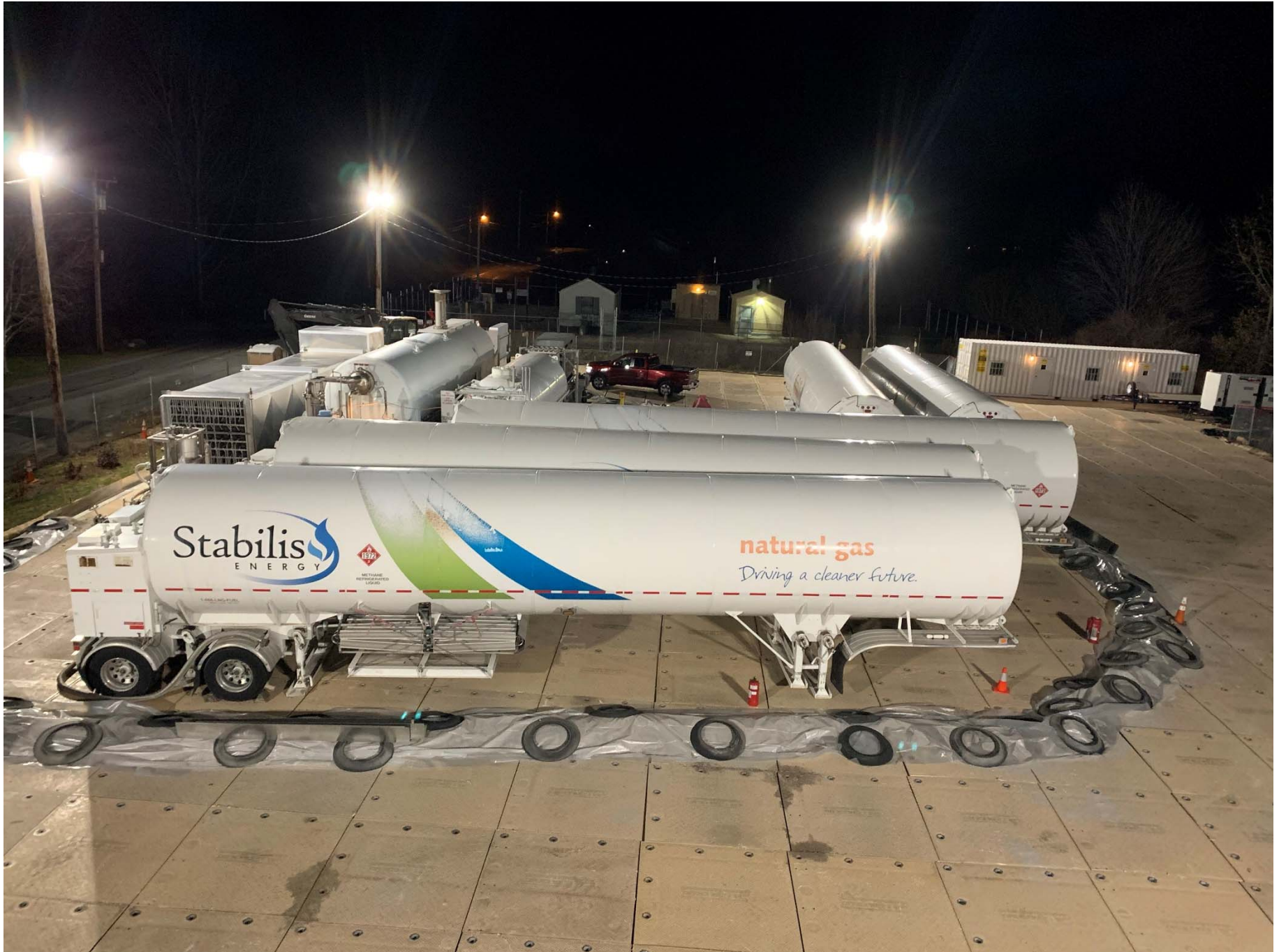
Exhibit D Photos of Installed Equipment (November 2019)
