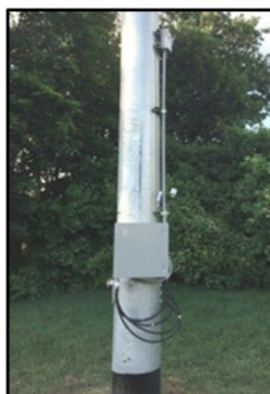
Figure 5.2: Substation / High-Capacity Network Gateways (109)
