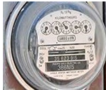
Electromechanical AMR Meter
