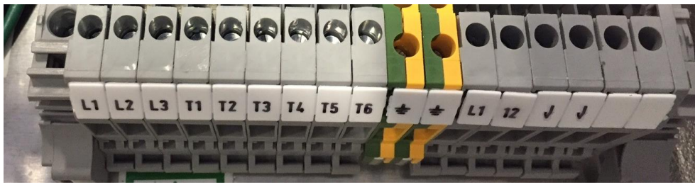
One-line wire diagram for installing a two-speed explosion proof blower motor. Diagram shows the wires from the motor to control and from thermostat to control. Terminal block image in the control is also shown for reference.
