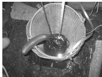
Pump and oil sensor supported inside filter basket.
