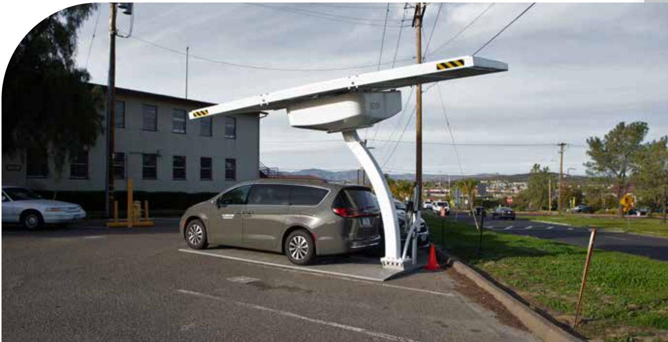
An electric van docks at a new solar-powered electric vehicle charging station on Marine Corps Base Camp Pendleton, CA. The self-contained, portable charging stations are independent from the electric grid, can be installed immediately, fit over a parking spot, and be moved to support mission essential tasks or be used during emergencies as a power bank, increasing overall mission resilience for U.S. forces. The Marine Corps' Southwest Region Fleet Transportation Office recently acquired two of these charging stations to add to their existing permanent electric vehicle charging infrastructure at Camp Pendleton, Jan. 12, 2022.
