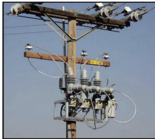
Figure 6.19: Recloser on a Distribution Pole
