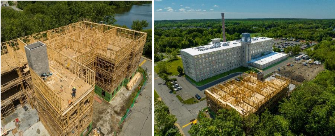
Images of Bourne Mill Phase 3 under construction are courtesy of Rhode Island Housing
