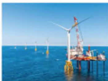
OPENING THE GATE: Deepwater Wind LLC completed the Block Island Wind Farm, pictured, in 2016. In June, the first utility-scale wind farm, an 84-turbine project called Vineyard Wind proposed off Martha's Vineyard, received a favorable preliminary analysis from the Bureau of Ocean Energy Management, paving the way for future wind farms to begin spinning. COURTESY DEEPWATER WIND LLC
