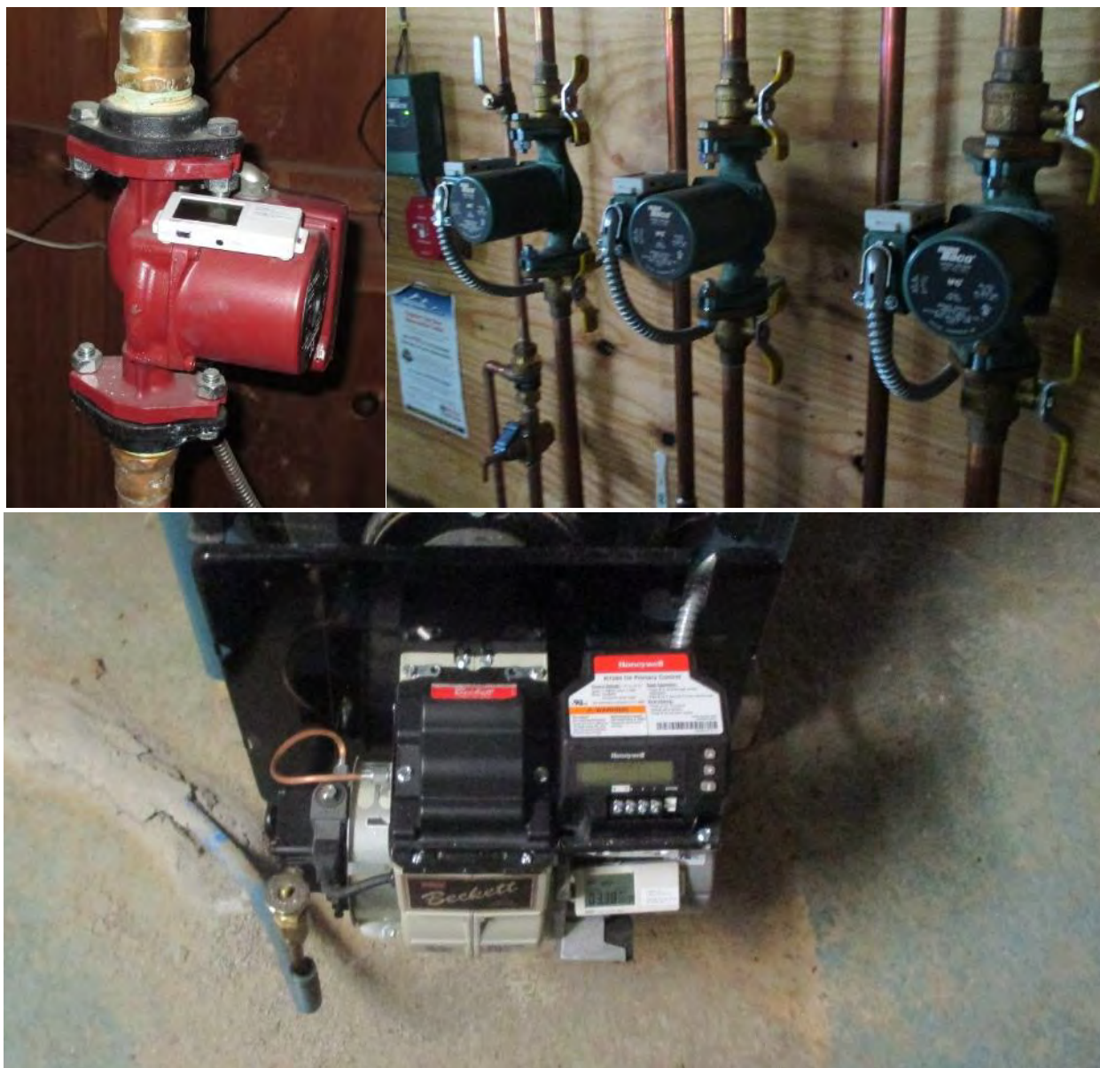
Figure 11. Boiler System Monitoring
