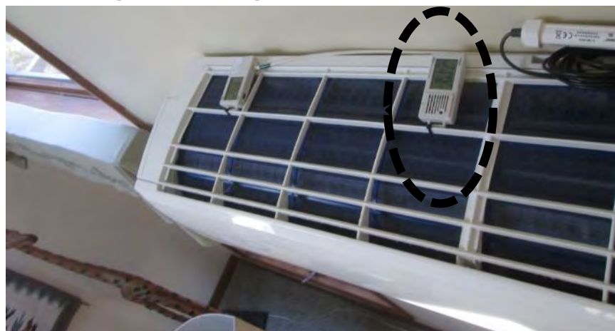
Figure 10. Entering Air Sensors on a DMSHP Head
