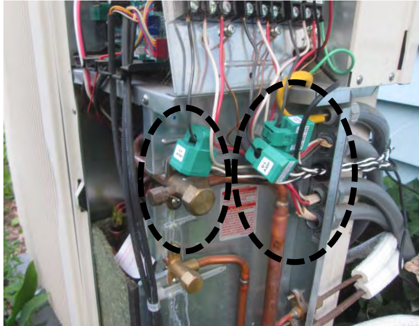
Figure 6. Current Transformers Installed on Fan Wires
