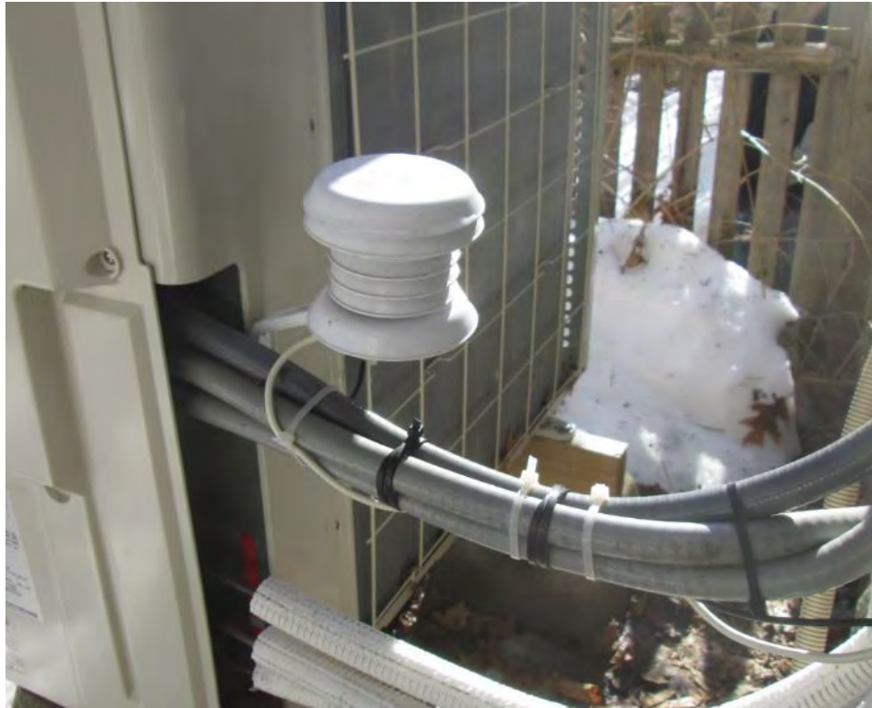
Figure 8. Outdoor Entering Air Temperature and Relative Humidity Sensor
