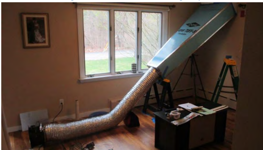
Figure 88. Powered Flow Hood Testing Setup
