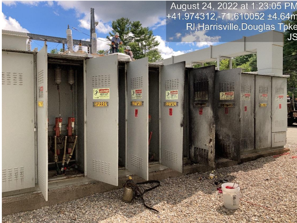
Illustration of what failed (Source RIE report dated November 16, 2022, additional picture in Appendix B)
