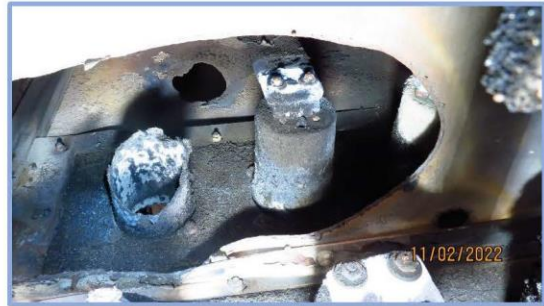
Rosette Insulating Tubes: View from Rear of Switchgear Note the breakdown of the left tube.
