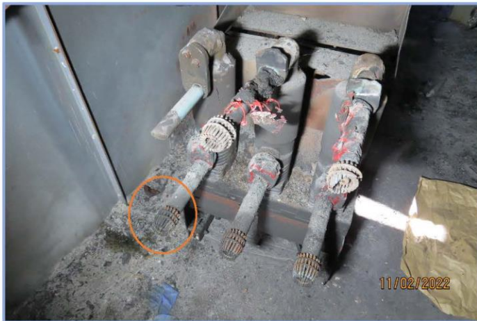
Failed 41 Feeder Breaker Showing Condition of the Rosettes Note: Top middle and right breaker conductor tubes have been reattached to show rosette positions. Note: Top left rosette completely burned from arcing.
