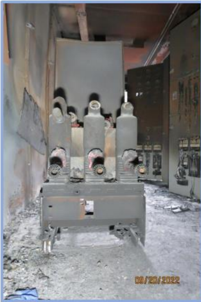
Failed 41 Feeder Breaker
