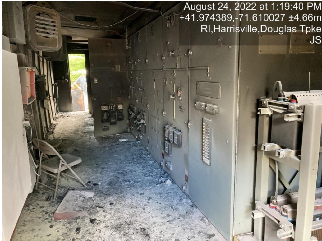
Below shows the fire damage to the inside of the station switchgear building, specifically the 41-breaker cell, dated August 24, 2022. The majority of the fire damaged occurred inside of this cell.
