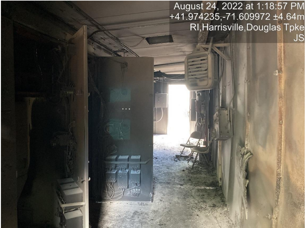
Below shows the fire damage to the inside of the station switchgear building, from the opposite end of the building than the picture above, dated August 24, 2022.
