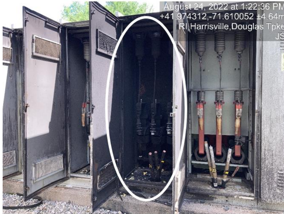
Below, shows the outside access to the 41-feeder breaker cell (left) which shows extensive fire damage and the far less damage to the neighboring breaker cell (right). Dated August 24, 2022.
