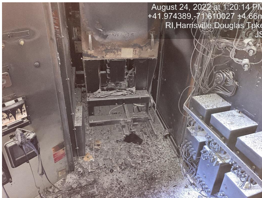
Below, the white circle, shows the outside access to the 41-feeder breaker cell which shows extensive fire damage.
