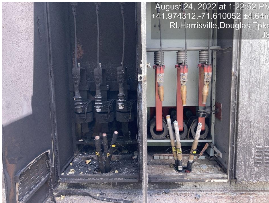
Below, shows the fire damage to the back of the station switchgear building, dated August 24, 2022.
