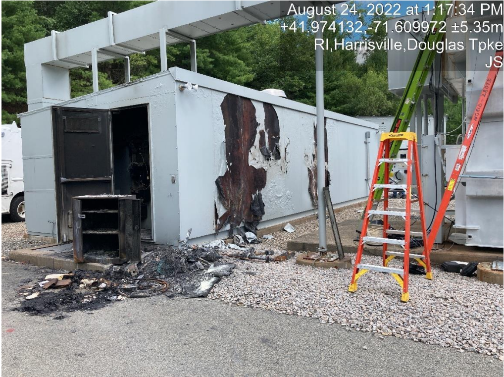
Below shows the fire damage to the inside of the station switchgear building, dated August 24, 2022.
