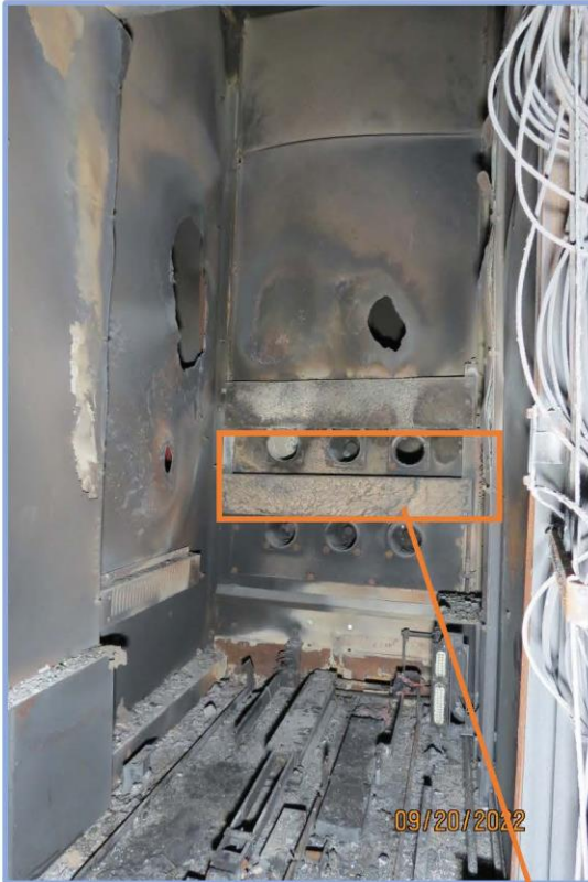
41 Feeder Switchgear Cell
