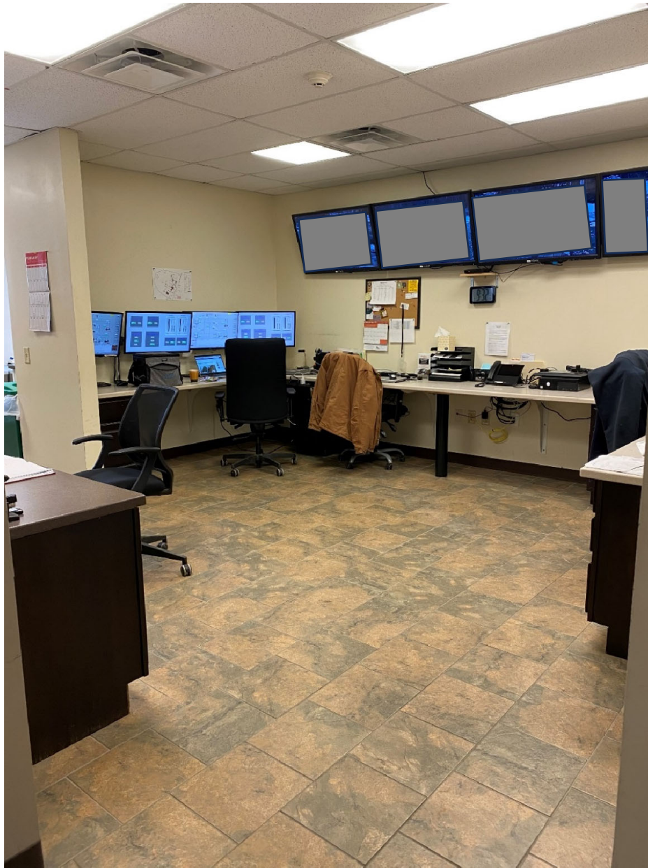
The picture above contains a view of security camera monitors for the Cumberland LNG site. The images on the security cameras have been grayed out for security purposes.
