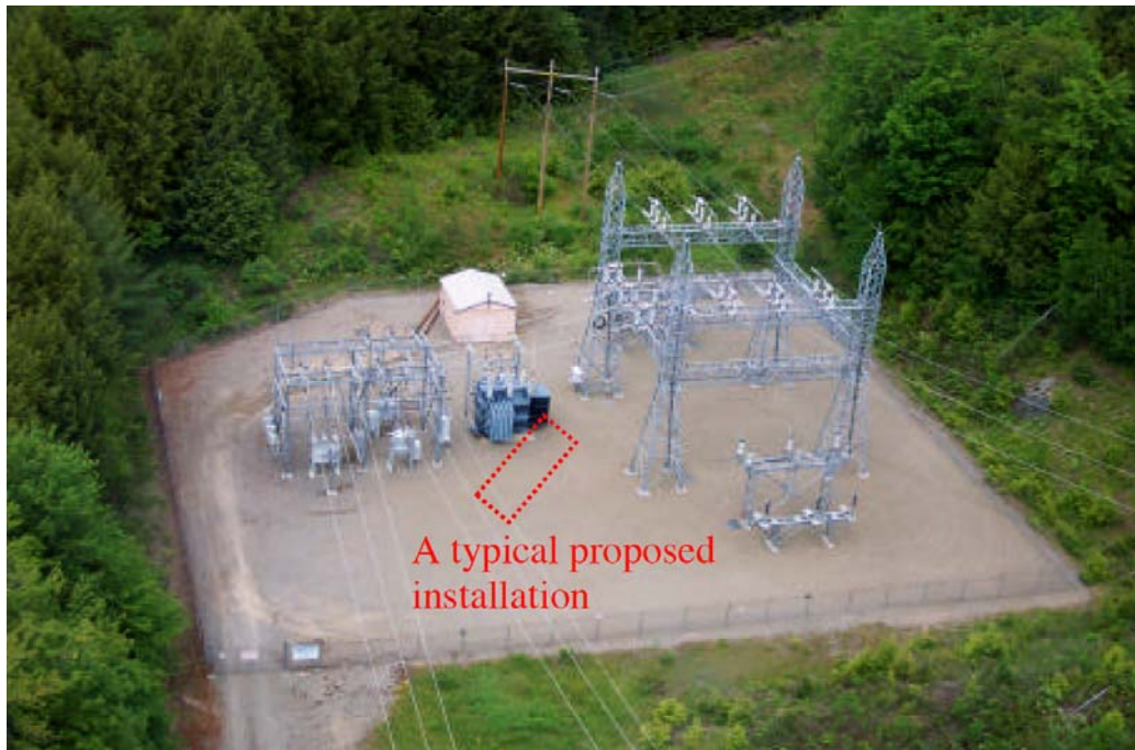
Fig. 10. MTS proposed position within Vermont Electric substation.
