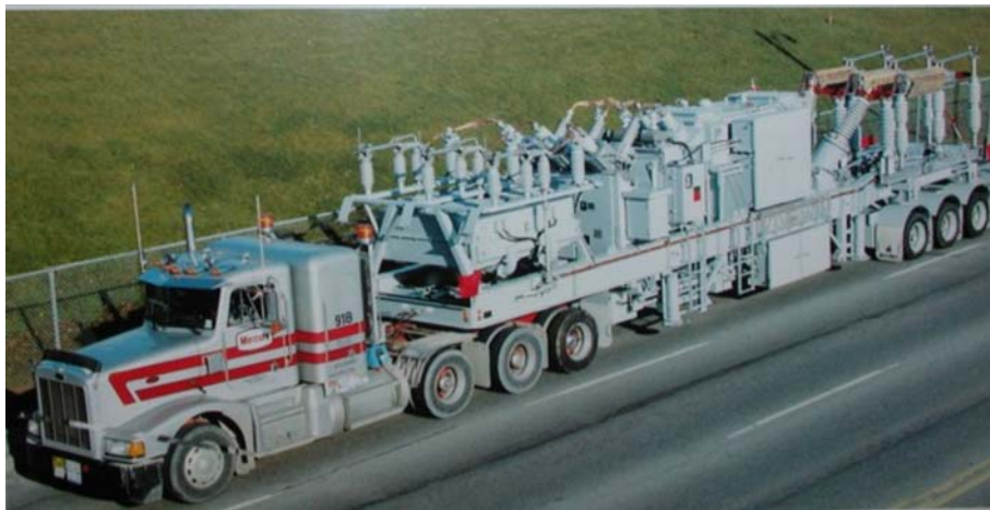
Figure 7. Mobile substation in transit.
