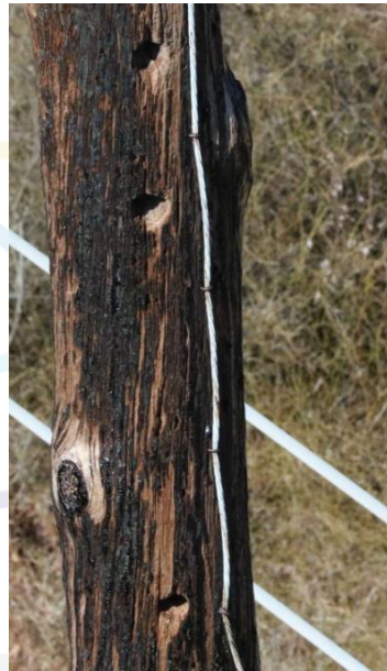
Woodpecker Damage on 332 Str 164 Wood H-Frame (1970)
