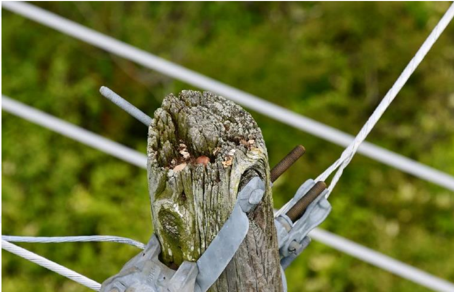
Heavy Pole Top Rot on 332 Str 39 Wood Monopole (1970)
