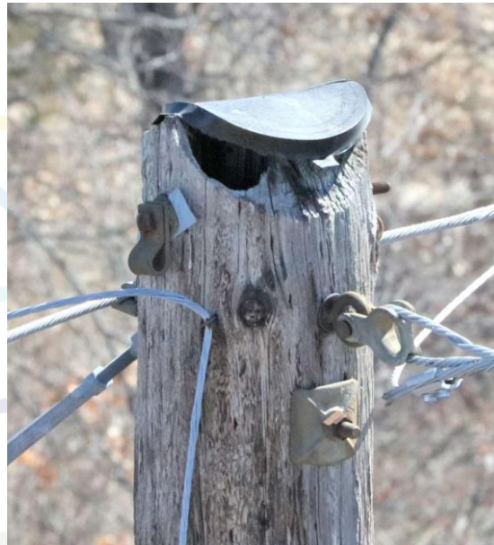
Pole Top Deteriorating on 332 Str 112 Wood H-Frame (1970)
