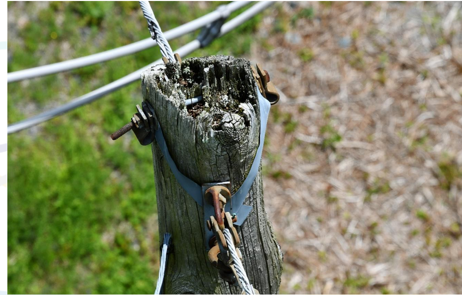
Heavy Pole Top Rot (Exposed Through Bolt) on Str 33 3 – Wood Pole (1971)
