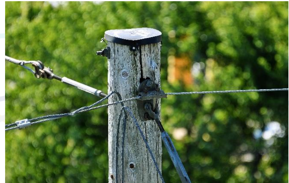
Pole Top Crack on 332 Str 129 Wood H-Frame (1999)
