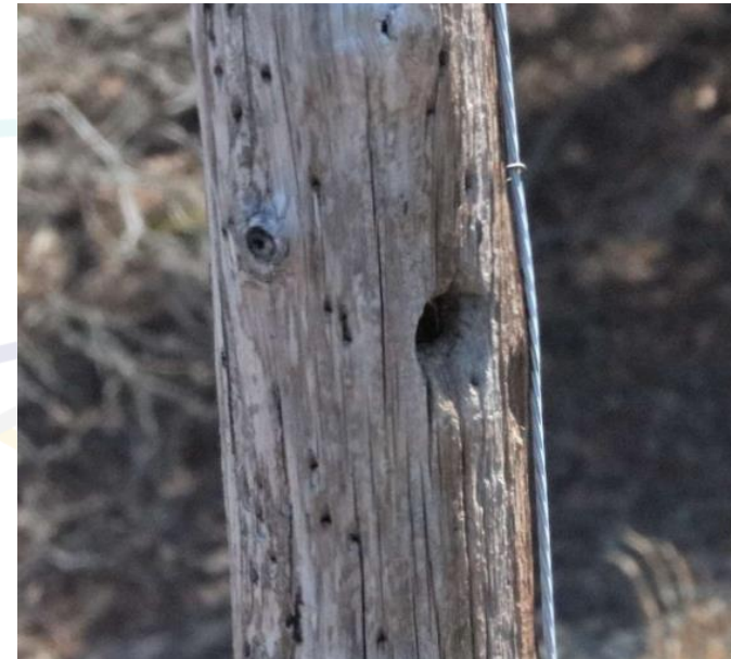
Woodpecker Damage on 332 Str 103 Wood H-Frame (1971)
