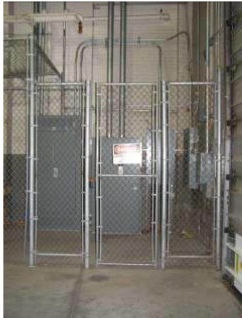
Providence Electrical Service
