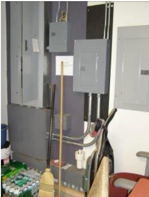
Cranston Electrical Panels
