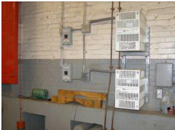
Providence Electrical Equipment
