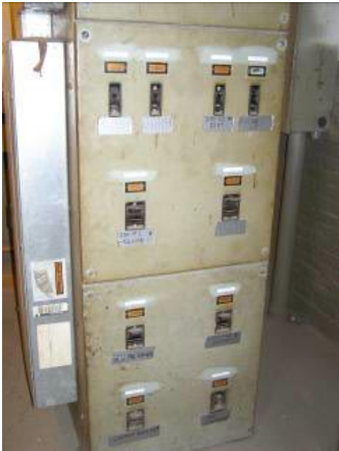
Providence Electrical Gear
