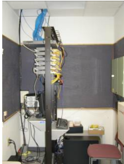
Cranston Server Equipment
