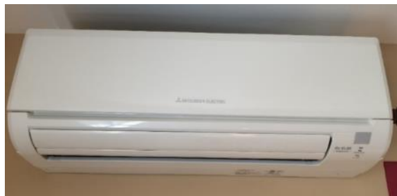
Figure 2. DMSHP Indoor Unit
