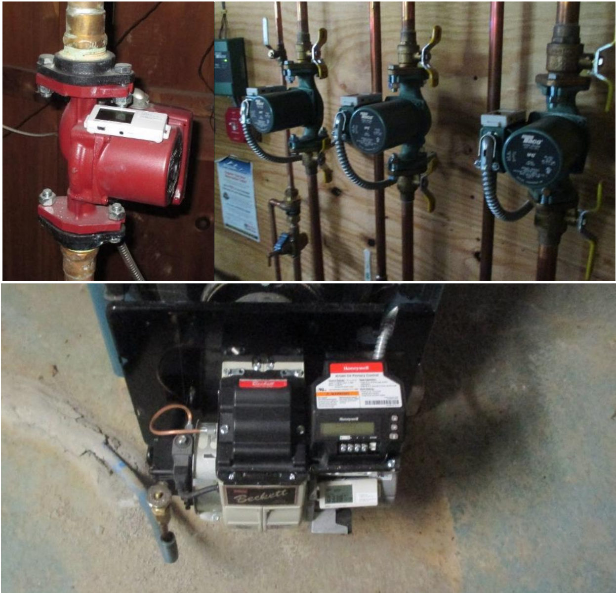
Figure 11. Boiler System Monitoring
