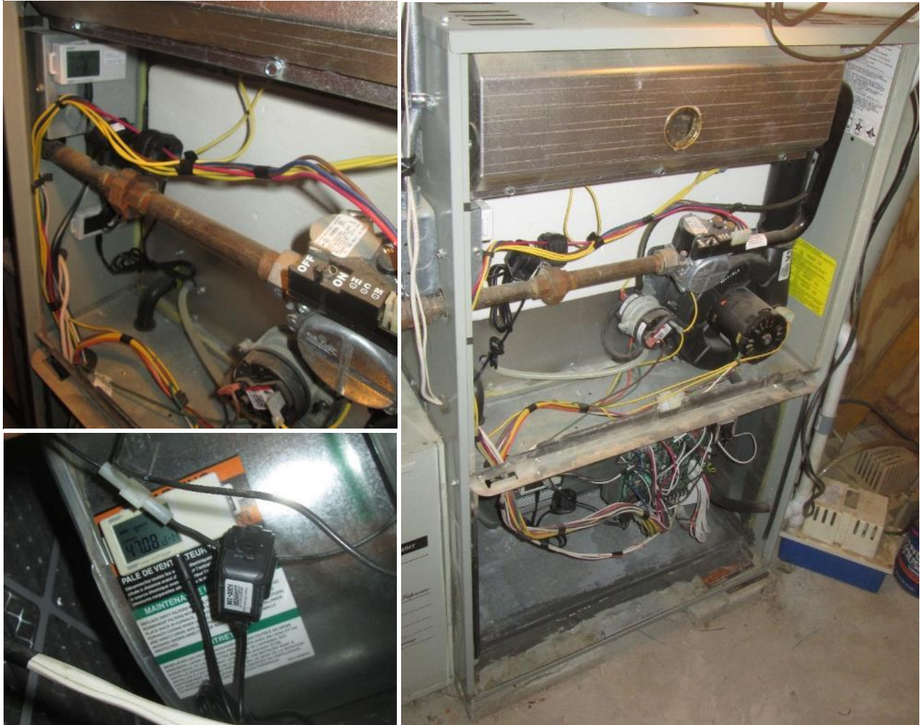
Figure 12. Furnace System Monitoring
