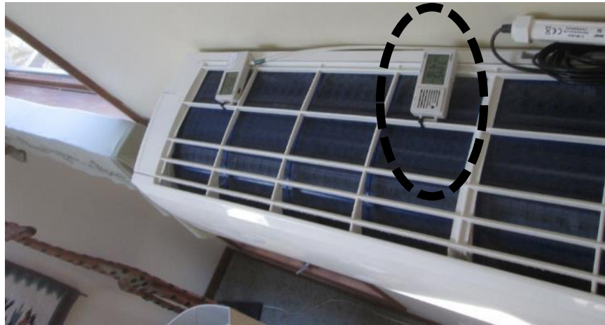
Figure 10. Entering Air Sensors on a DMSHP Head
