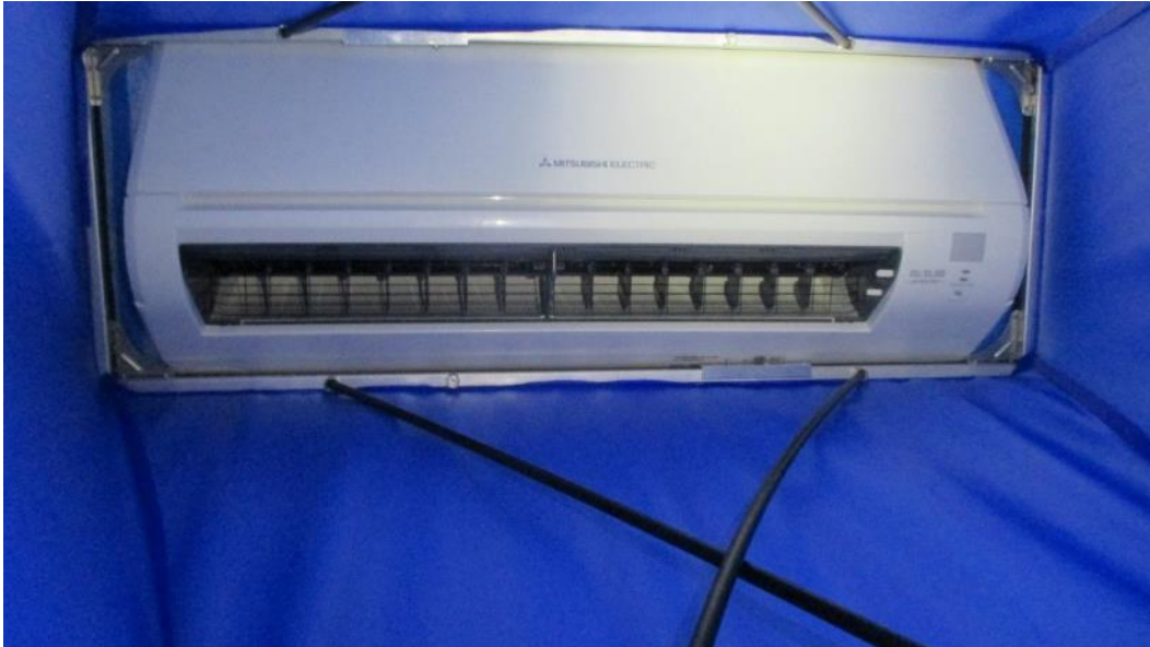
Figure 93. Non-Powered Flow Hood (Balometer) Setup
