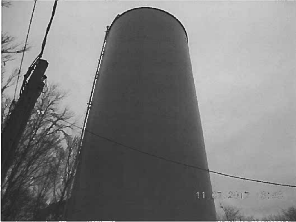
Account 330, Distribution Reservoirs and Standpipes Tank - Standpipe
