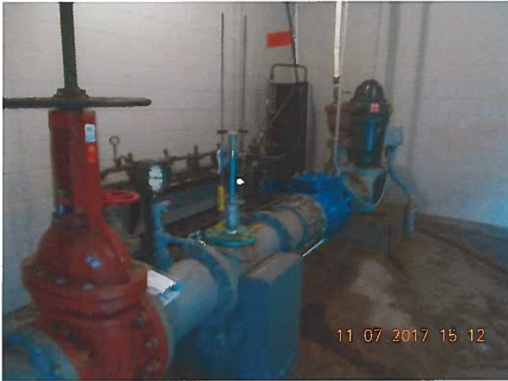
Account 307, Wells and Springs Wellhead
