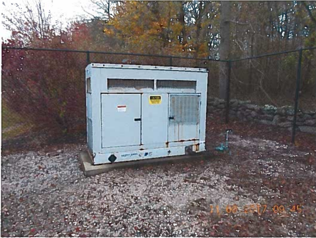
Account 311, Electric Pumping Equipment Generator
