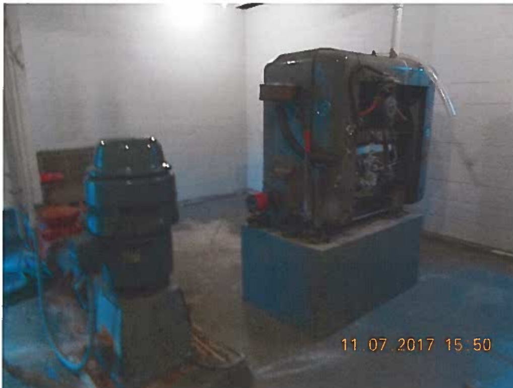
Account 311, Electric Pumping Equipment Pump and Motor
