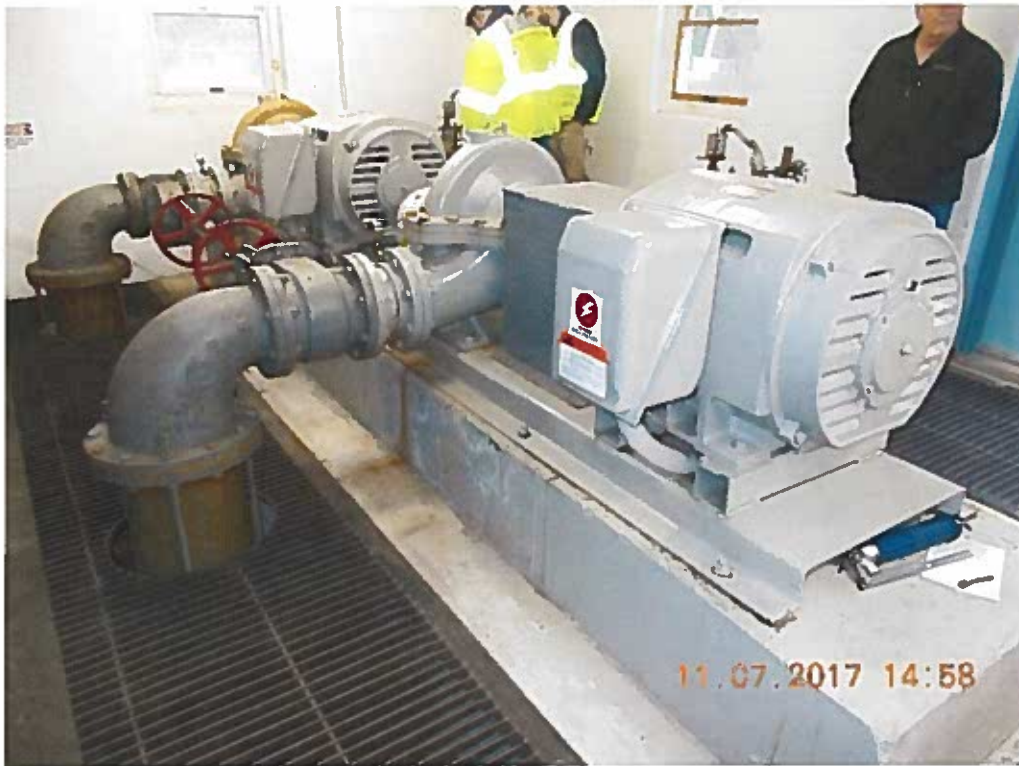
Account 311, Electric Pumping Equipment Two Pumps #2 & #3
