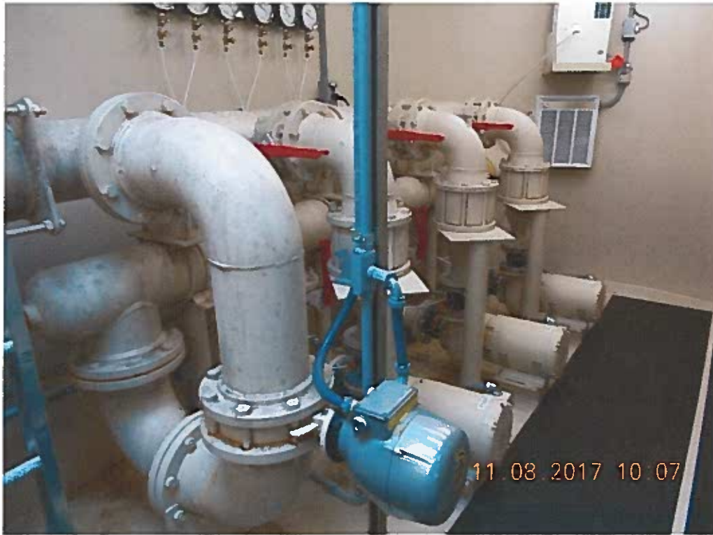
Account 311, Electric Pumping Equipment Pumps
