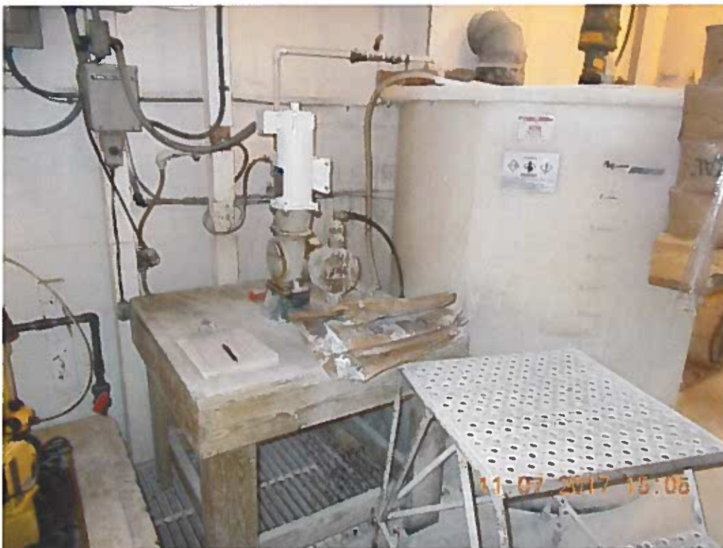
Account 320, Water Treatment Equipment Lime Slurry Equipment
