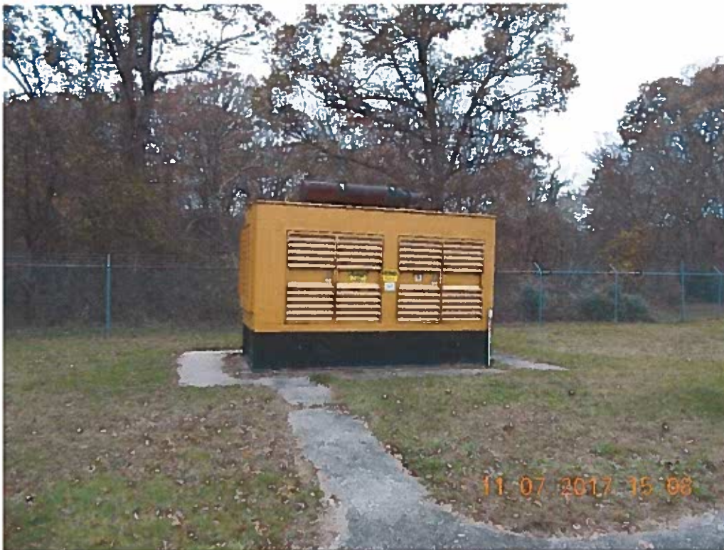
Account 311, Electric Pumping Equipment Emergency Generator
