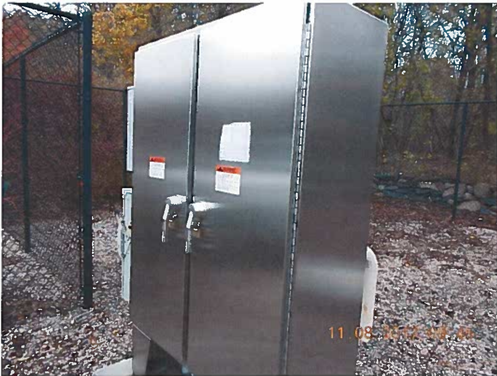
Account 311, Electric Pumping Equipment Electronic Panel
