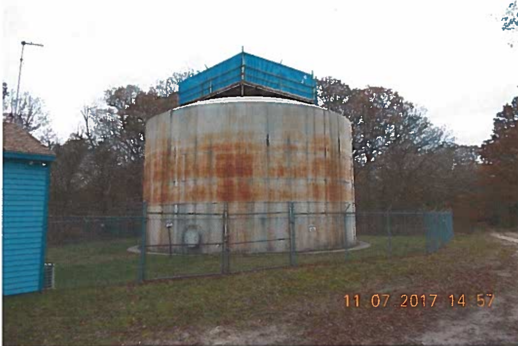
Account 330, Distribution Reservoirs and Standpipes Standpipe and Air Stripper
