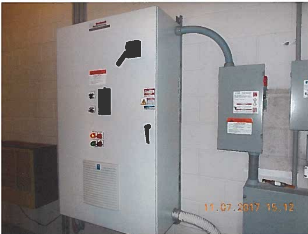
Account 311, Electric Pumping Equipment VFD
