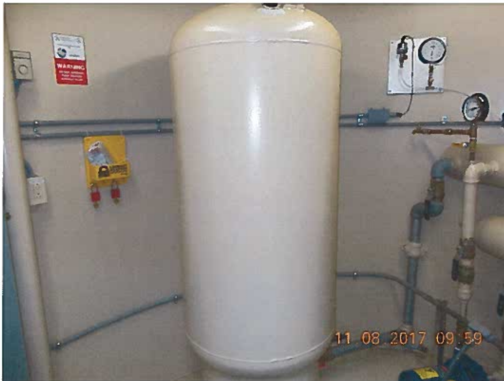
Account 311, Electric Pumping Equipment Pressure Tank
