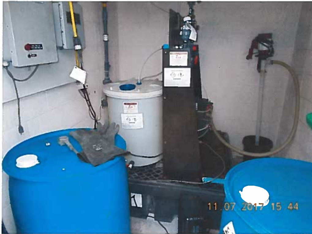
Account 320, Water Treatment Equipment Sodium Hypochloride
