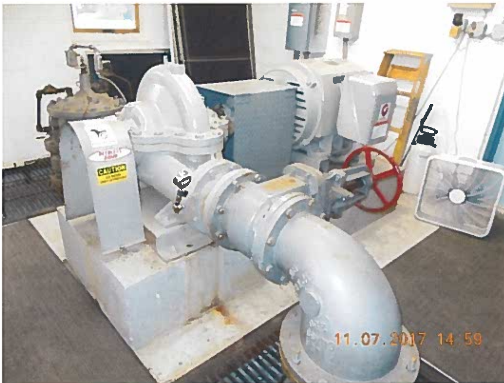
Account 311, Electric Pumping Equipment One Pump – 150 HP
