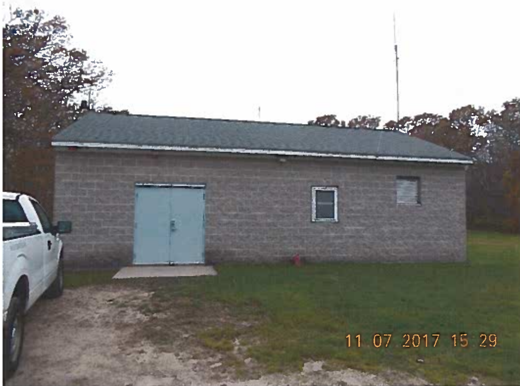
Account 304.1, Structures and Improvements - Source of Supply Booster Building
