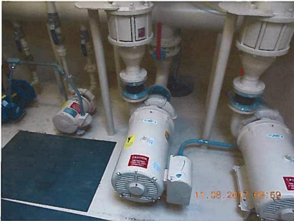
Account 311, Electric Pumping Equipment Pumps
