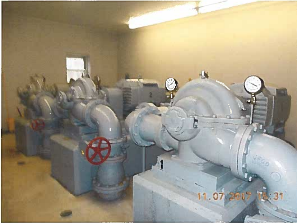
Account 311, Electric Pumping Equipment 3 Booster Pipes – 200 HP
