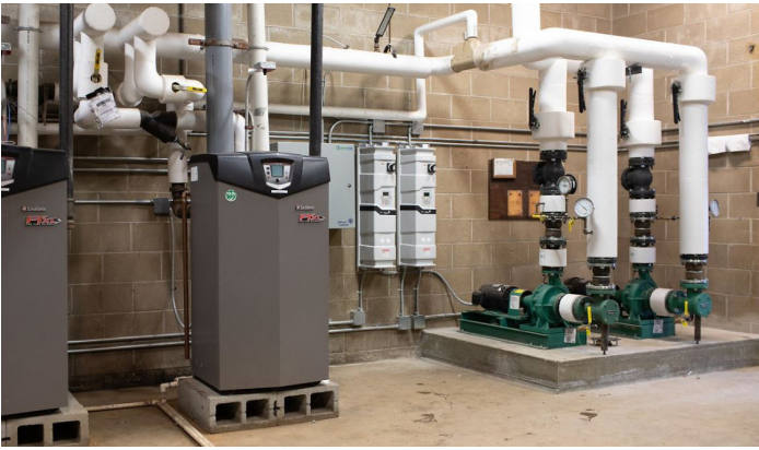
The City of Pawtucket's investment in building management systems helped to significantly reduce energy costs.
