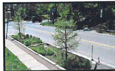
Stormwater Raingarden Bump Out
